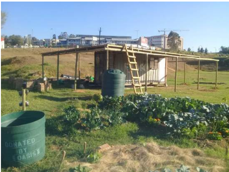
Construction is nearing completion on the container and storage unit at the Agroecology Training and Demonstration Centre.
